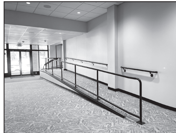
A new handicap ramp with a gradual slope replaces the makeshift ramp which had previously been used to go up a short flight of four stairs. According to ADA guidelines, with every inch of vertical rise, a ramp must be 12 inches long.
